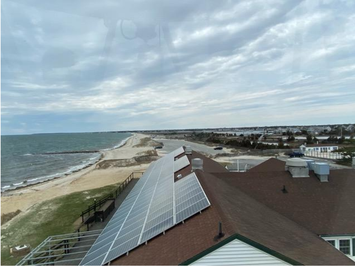
Solar panels were installed on three buildings at the Lighthouse Inn. View looking westward towards West Dennis Beach.
